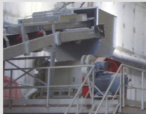
Russia – Pre-roller mill and fine roller mill
